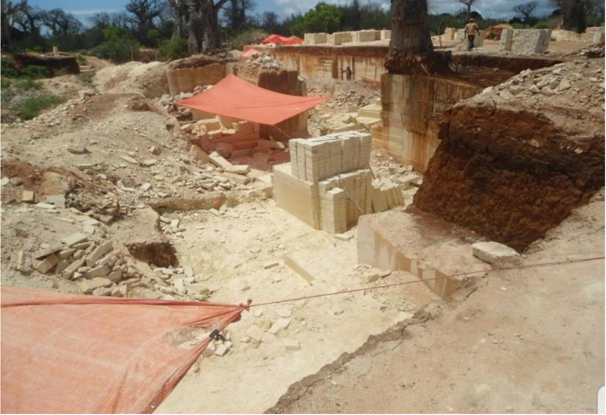
The top view of the Micheweni manual stone crushing site where the tent is used for sun burn protection (source researcher 2021)
